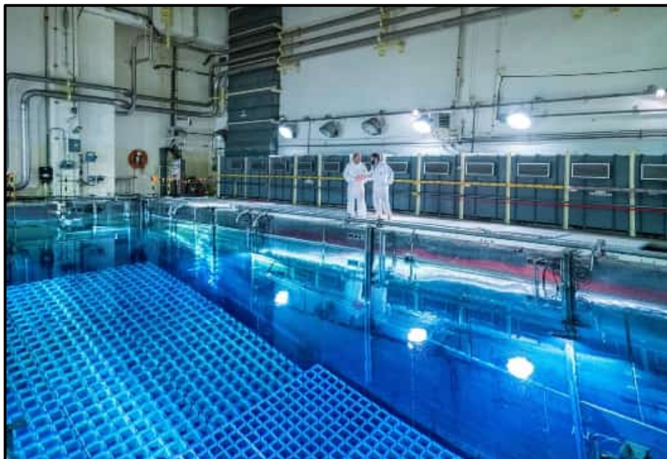
Spent fuel pool Nuklearna elektrarna Krško. "Spent Fuel Pool." https://www.nek. si/en/how-nek- works/spent-fuel- pool
